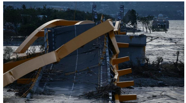
Collapse of Palu Bridge IV due to earthquake shaking
